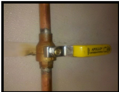
Shut Off Valve
